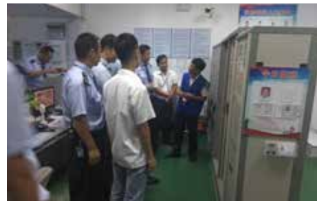
Fire safety panel training
